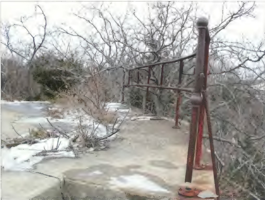
Figure 3.10. View of guardrail south of emplacement #1, Battery Peck. The railings are in fair to poor condition with corrosion covering most pieces. Some assemblies lack any solid material where the vertical members fasten the railing to a solid support (Olmsted Center, January 2009).
